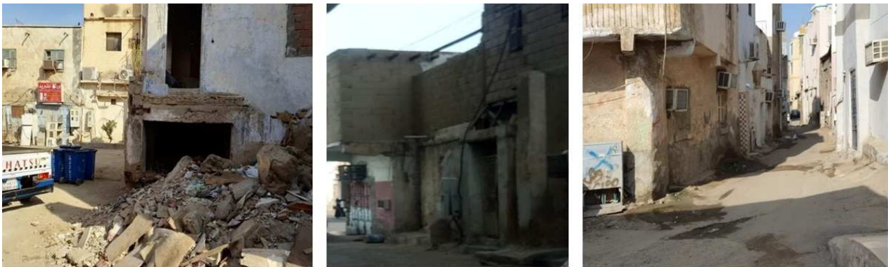
Fig. 7. Examples of buildings with deteriorated physical condition.
