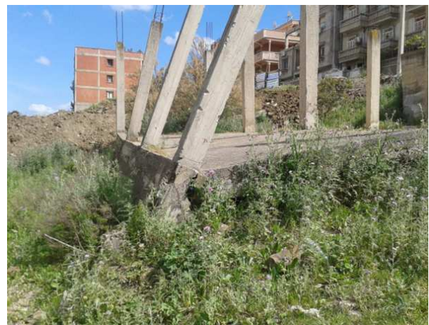
Fig. 9. Unregulated expansion of informal individual housing beyond the urban development zone, alongside the risk of sliding in the area.
